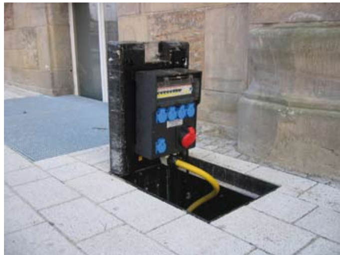
Completed installation of the CAMPETTO
